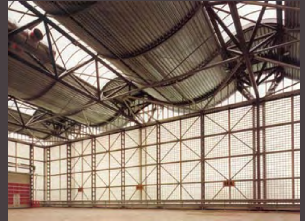
Overslagstation AVR, Jan Brouwer Associates
